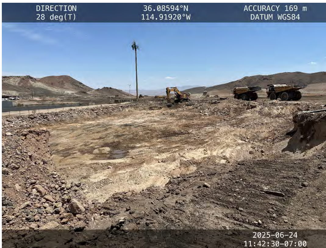
Tailings seam southeast of Tailings Pond 1 – June 24, 2025
